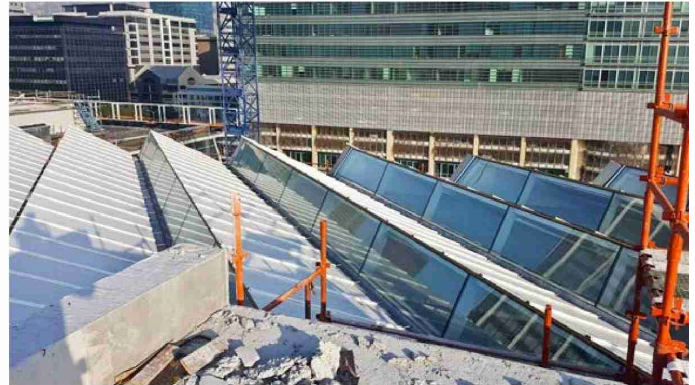
CTICC East The saw-tooth structure was kept as light as possible using tubular sections to keep the roof space uncluttered
